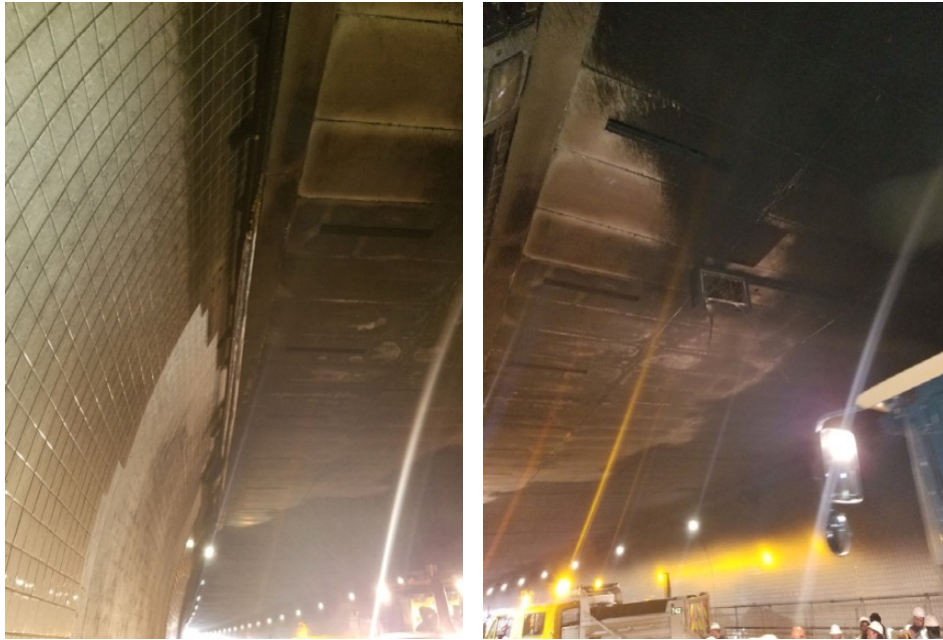
Figure 8 - Lifeline® RHW-2 in FRE Composites XW BreathSaver® Phenolic conduit, installed along the length of the tunnel, remained operational throughout the fire event 5
